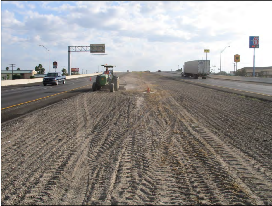
Figure 1.1. Seeding a Recently Completed Right of Way along US HWY 77 in South Texas.
