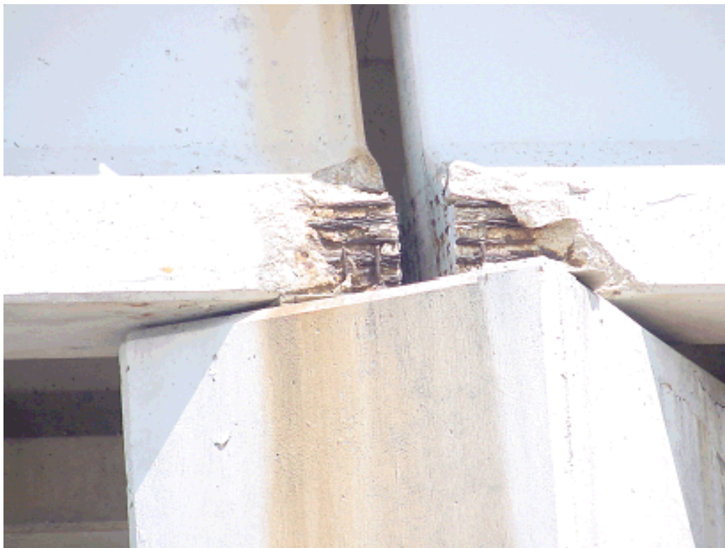
Figure 9-5. Chemical Solution Corrosion Induced Beam Damage Created by Failed Joint and Poor Concrete Cover over Beam Ends.
