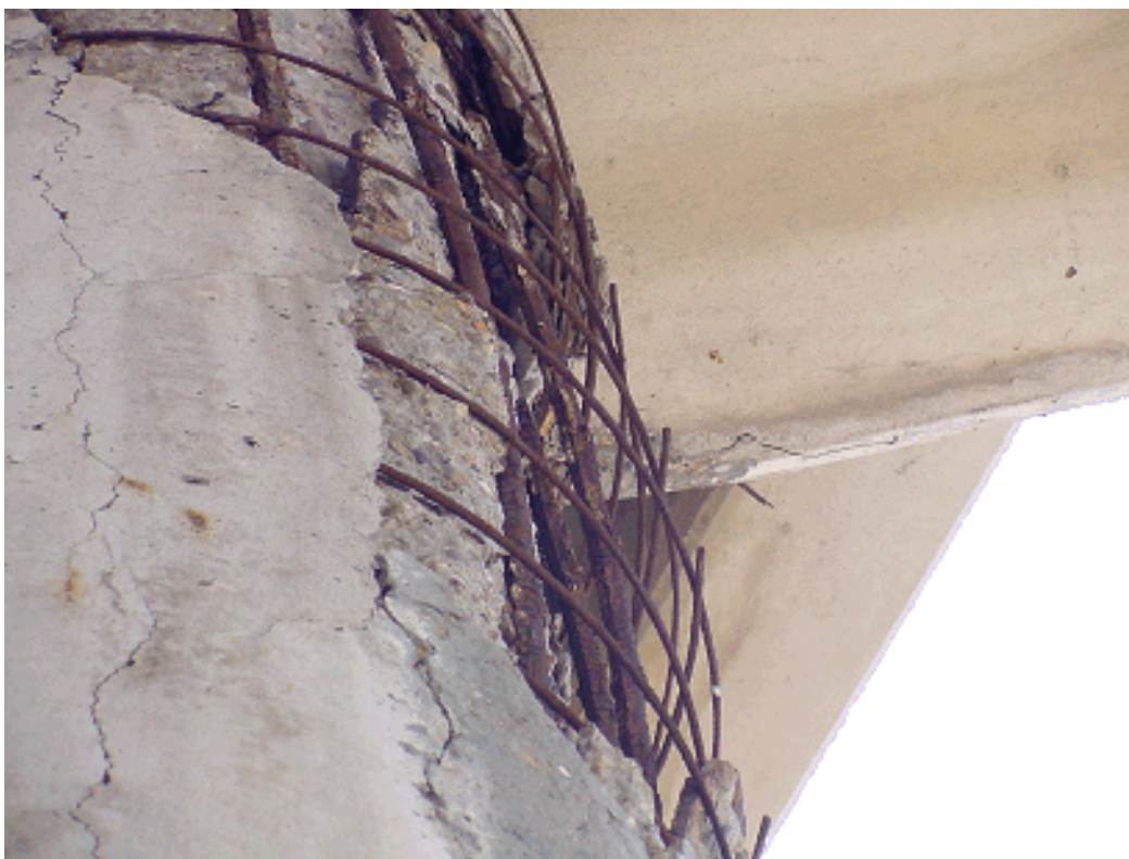
Figure 9-10. Close up of the Damage. Notice the #9 bars Are Starting to Buckle. Two Reasons This Could Be Happening: (1) Rust Could Be Pushing on Concrete Causing the Buckling. (2) The Column Could Be Shortening. This Bridge Was Replaced after 20 Years of Service.
