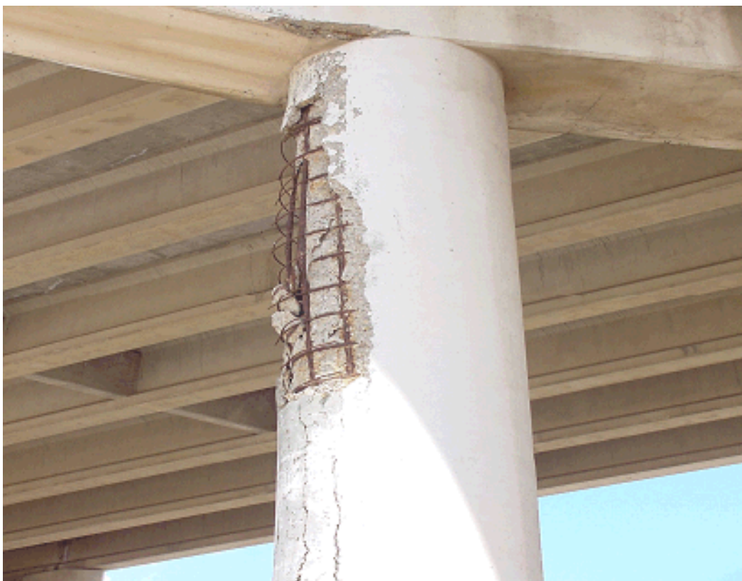
Figure 9-9. Column Deterioration from Chemical Solution Contamination.
