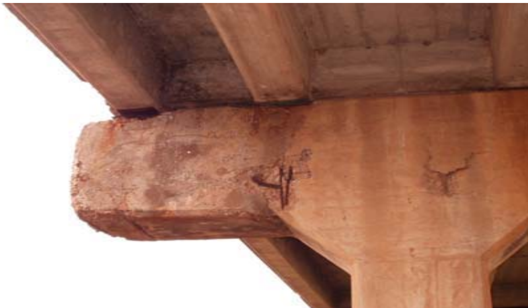
Figure 9-7. Corrosion Induced Damage in High Stress Cantilever Design.
