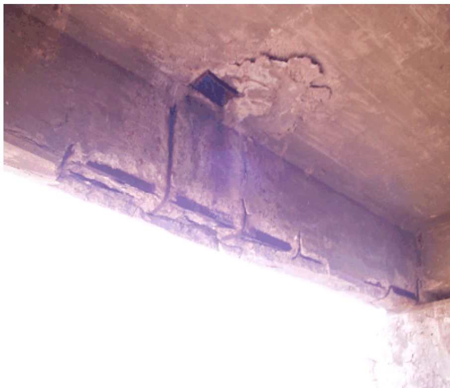
Figure 9-1. Corrosion Damage due to Concentrated De-icing Solution at Drain Site.
