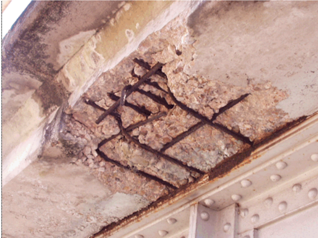
Figure 9-4. Poorly Maintained Joint Allowed De-icer Solution to Damage Overhang to Second Mat of Steel and Top Plate Steel on Beam.
