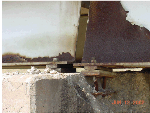
Figure 9-8. Failure on Cap due to Corrosion Damage. Bridge Was Closed until Repair Could Be Performed.
