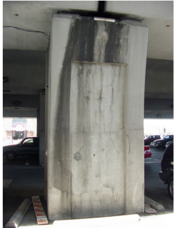
Concrete column affected by delayed Ettringite formation
