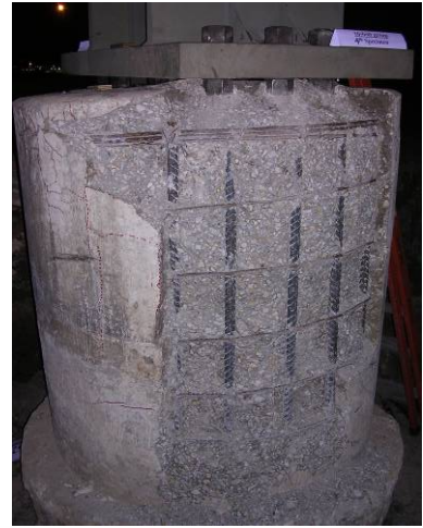
(c) After failure
