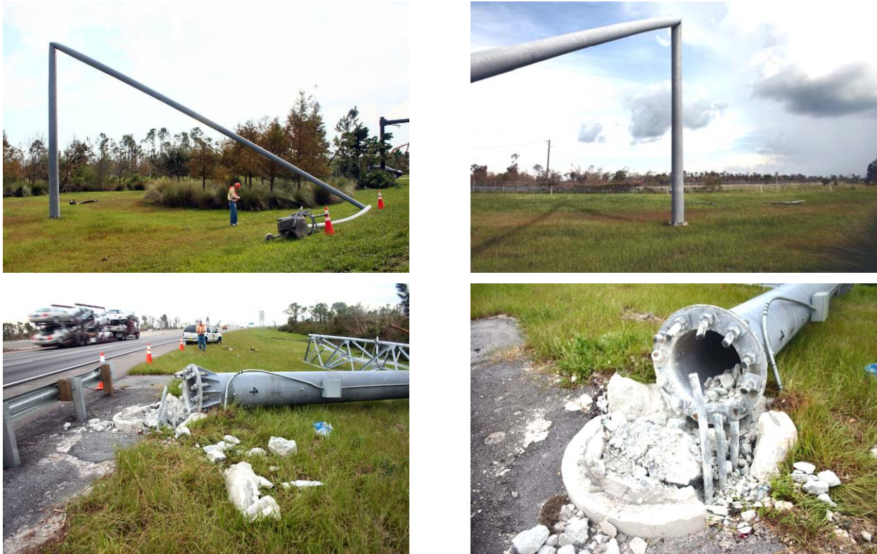
Figure 1.2 Failure of HMIPs and their Foundations (courtesy of Florida DOT)
