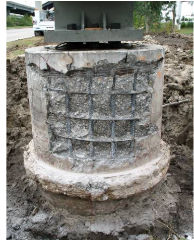
(c) After failure
