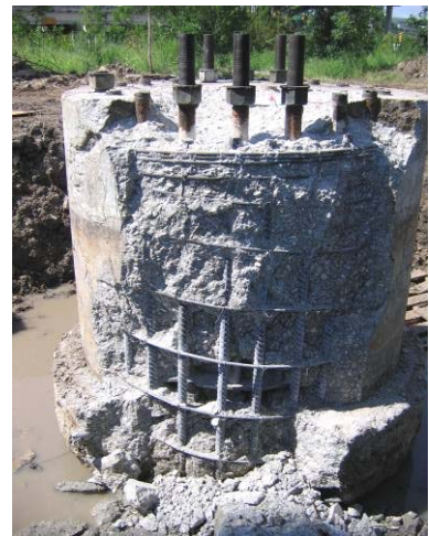
(c) After failure
