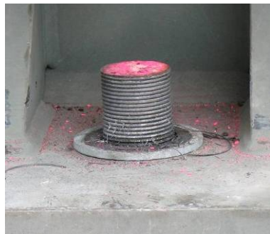
(a) Bolt Thread Stripping
