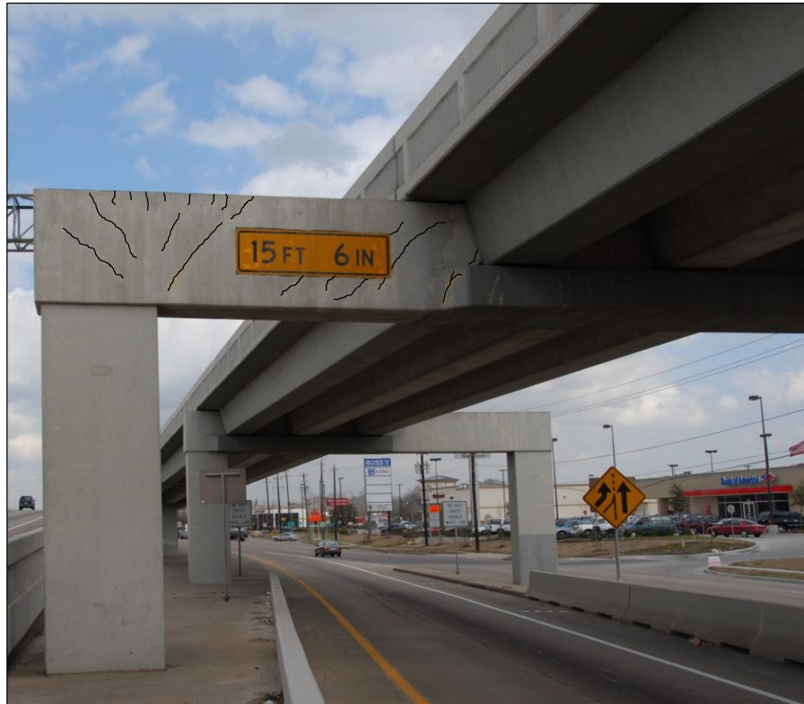
Figure 5-14: Diagonal Cracking within an Inverted Tee Bent Cap
